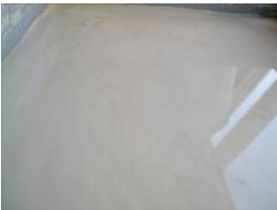
Figure 27: Remaining water a 1 cm deep
